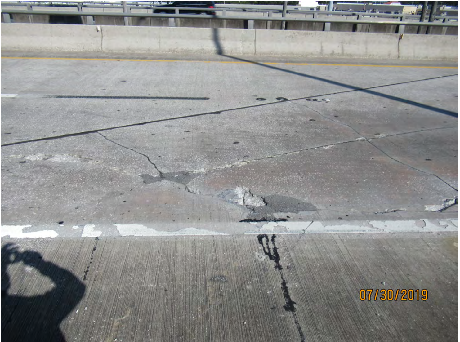
Photo 5: Element 321 Re Conc Approach Slab
