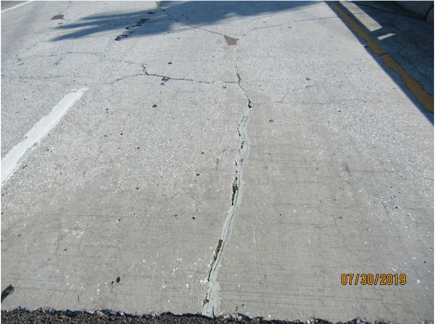
Photo 3: Element 321 Re Conc Approach Slab
