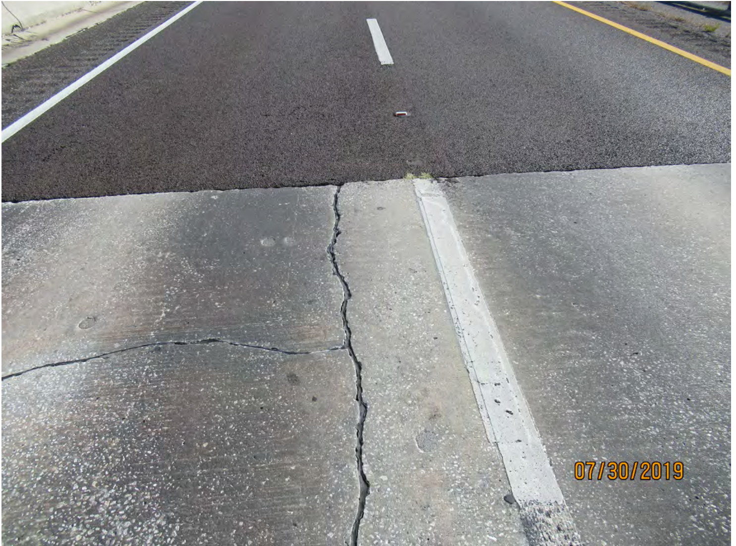
Photo 5: Element 321 Re Conc Approach Slab
