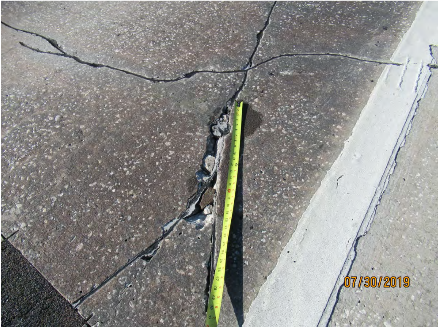
Photo 6: Element 321 Re Conc Approach Slab
