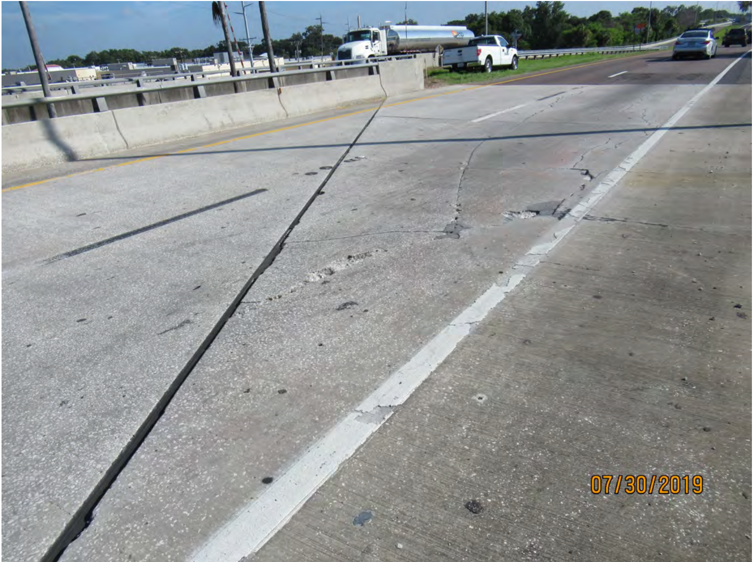
Photo 4: Element 321 Re Conc Approach Slab
