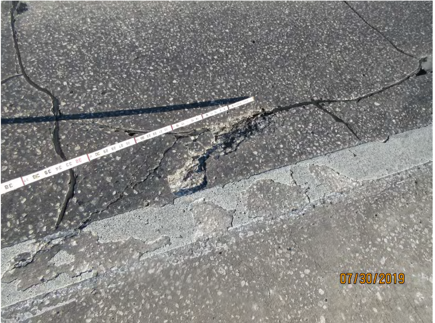
Photo 3: Element 321 Re Conc Approach Slab
