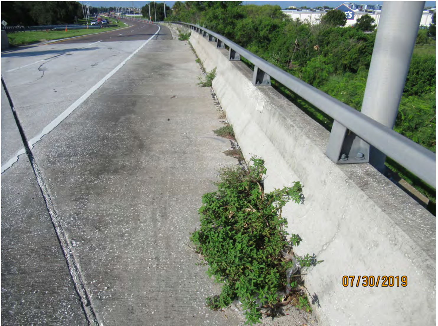
Photo 4: Element 321 Re Conc Approach Slab
