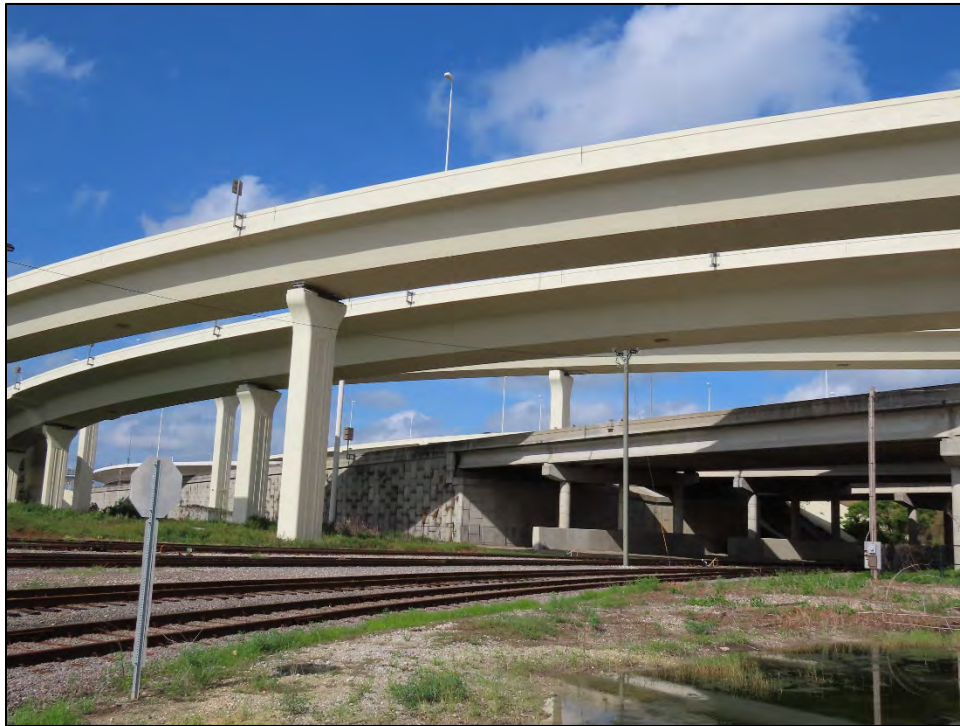
Figure 1: The Tampa Northern Railroad Gary Shops Spur (8HI15055) where it passes under the Selmon Expressway, facing Northwest
